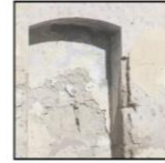
D: The door of church is blocked by bricks. It may be built after WWII.
