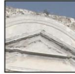
B: Carved stone is used as a decoration on the head of door. It was damaged to some extent.
