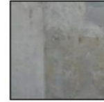
G: This part may be built with bricks after WWII, partially damaged now.
